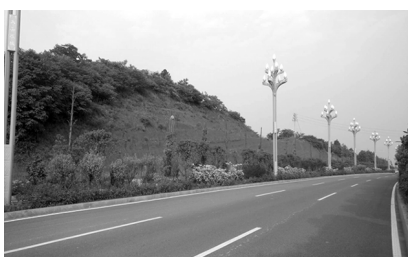
图 4 区域内某道路裸露边坡 Fig.4 A bare slope of a road in the area
